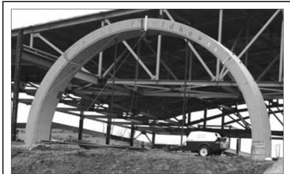
The soaring entry arch that will frame the main event entrance to the Richard and Helen DeVos Fieldhouse has taken its place on the building's east side. The arch stands 28 feet tall and 53 feet wide, and weighs 198,000 pounds. Made of post-tension, pre-cast concrete, the arch arrived in six pieces by truck and was assembled on-site. Construction continues throughout the winter on the building, scheduled to open in the fall of 2005.
