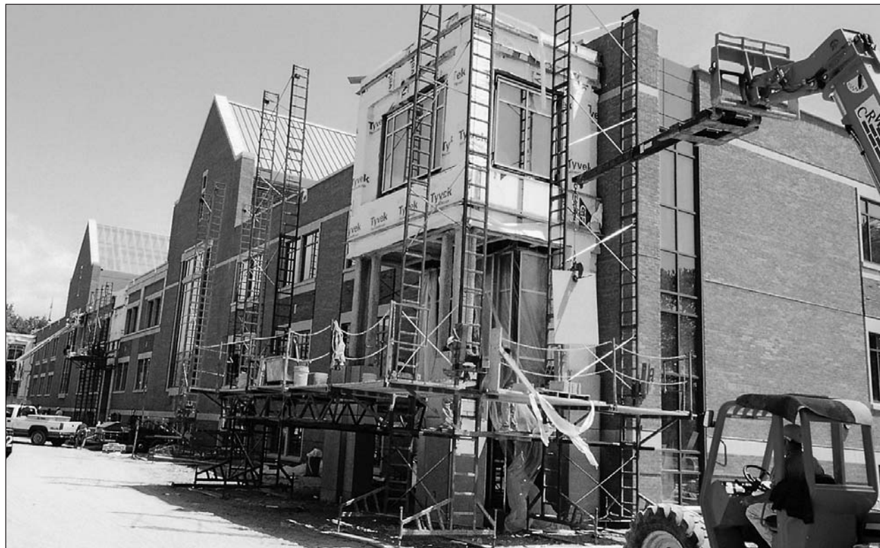
The exterior of the science center is well along as the August opening of the building approaches. A major challenge grant from The Kresge Foundation of Troy, Mich., will help fund the building—but only if other members of the Hope family provide additional support of their own.
